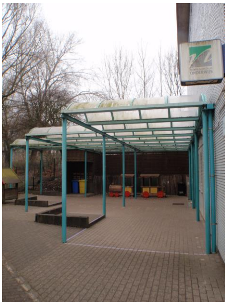
Photo 12 – PREAU A DEMOLIR
